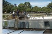
The construction of the home demanded a month and was transported to the lake in assembling parts.
