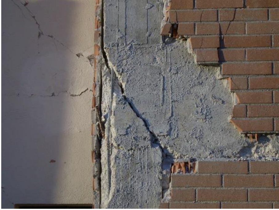
Figure 2.6. L'Aquila-Italy Earthquake (2009), Photo credit: Özgür AVŞAR [14]
