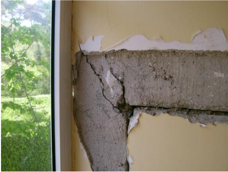
Figure 2.7. Simav-Turkey Earthquake (2011), Photo credit: Özgür AVŞAR [14]
