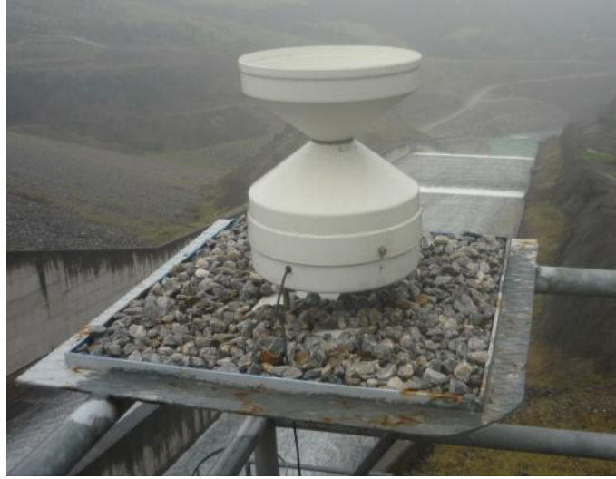
Figure 3.7 Rain-gauge (RG-6) located near the spillway without a heater (178 m)
