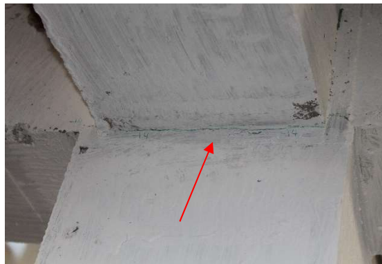
(a) First flexural crack in the columns
