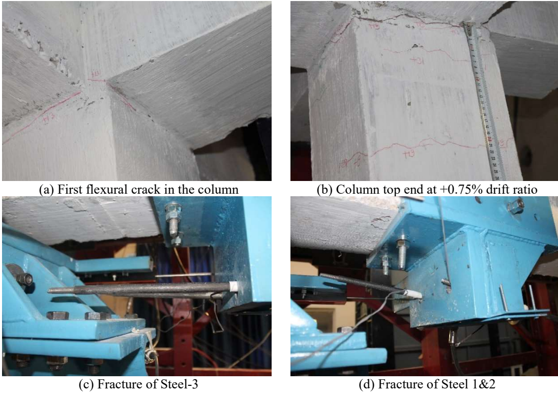
Figure 4.7. Failure pattern of G1-2-Steel at critical roof drifts
