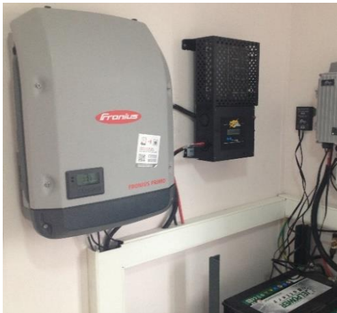
Figure 4. (a). On-grid Inverter (Fronius)
