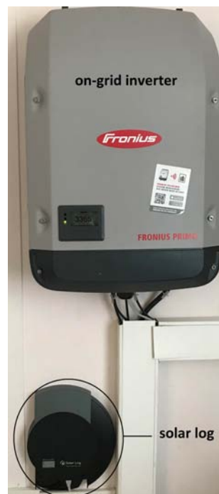
Figure 4. On-grid inverter with solar log.
