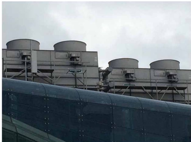
Figure 1 | Open recirculating CTs.
