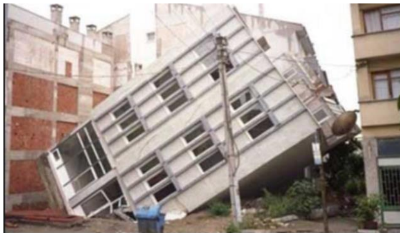
Fig. 1: An example of liquefaction damage.
